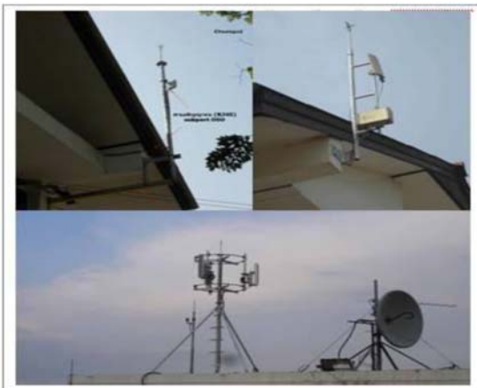
Fig.17:: The 3-sectors WBBNs antenna at Health center and MSMC building.
